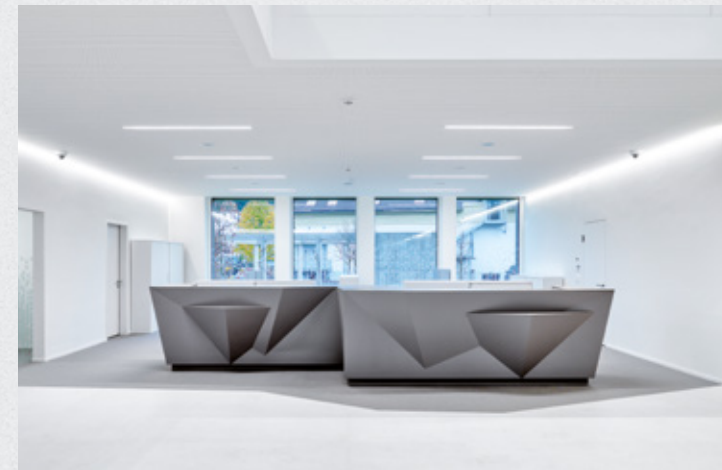
Clientis Bank Oberuzwil CH, In-ceiling sound system with DE Series speakers
